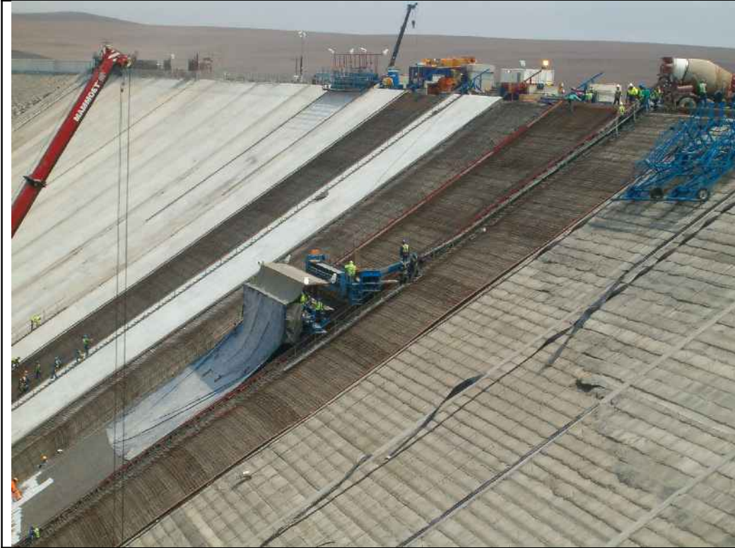
Bedford Dam Closer view of construction of upstream reinforced concrete membrane, on top of concrete kerbs at the outer edge of placed rockfill.
