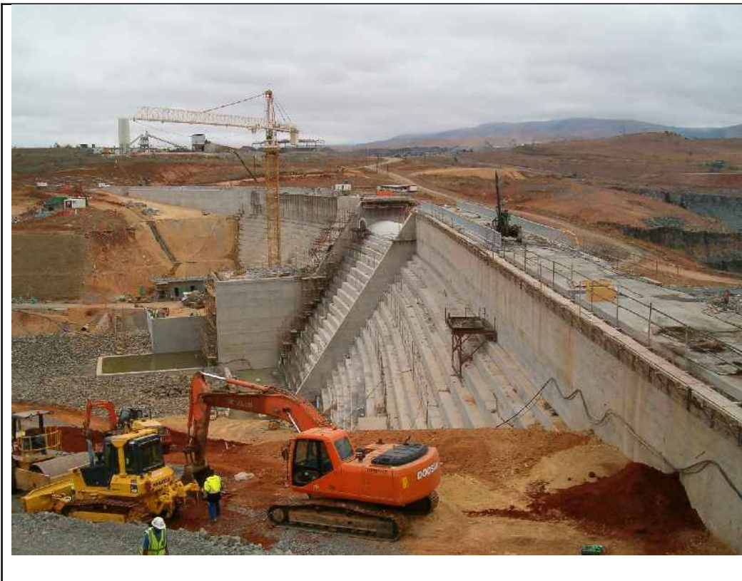
Bramhoek Dam (gravity arch) under construction near Ladysmith in KZN. ESKOM (Ingula Hydro Power Pump Storage Scheme). This RCC (roller compacted concrete) dam wall is also nearing completion, Sep 2010. This dam forms the bottom reservoir of the pump storage scheme.
